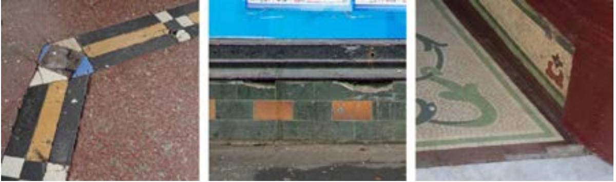
Damage to original tiling can often be easily repaired.
