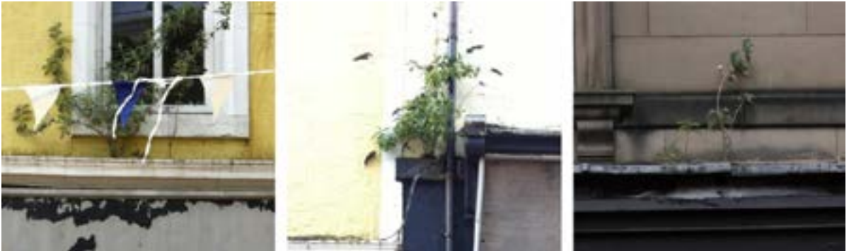
Vegetation growth allows water to penetrate into the shopfront, causing damage.
