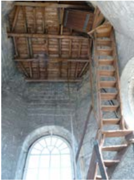
Interior of the Steeple looking up the stairs leading to the clock tower.
